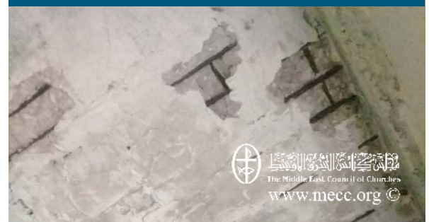
Another photo showing the status of ceiling in one of the visited buildings. The photo also shows that the building is not safe.
