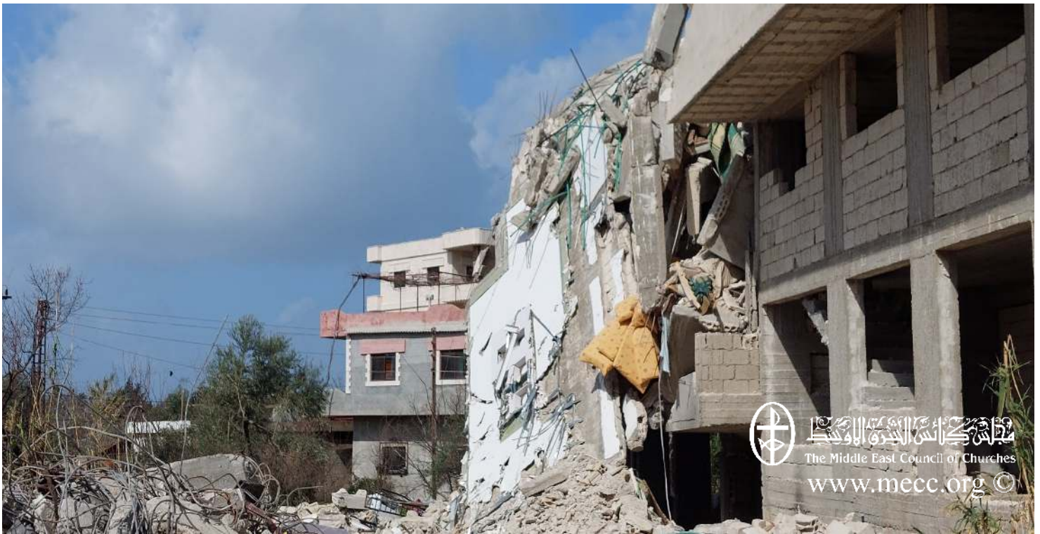
One of the affected Buildings in Jableh /Lattakia
