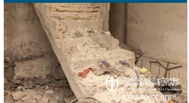
Status of one of basement of one building where the beams that link the foundation needs reinforcement
